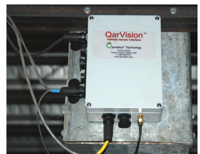
Machine room monitor installed in machine room
