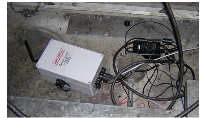
QarVision™ placed on top of elevator car
